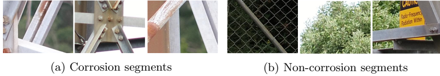
Figure 5: Example of Corrosion and non-corrosion segments
